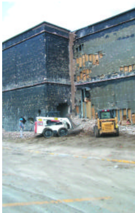
The Graduate School of Biomedical Sciences as brick is being removed at the beginning of the deconstruction process
